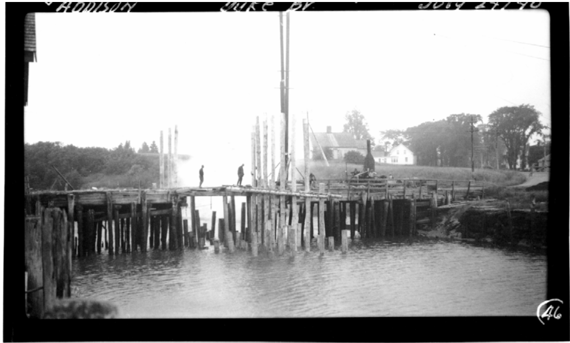
A steam powered hammer was used to drive pilings 35 feet down into the mud. July 24, 1940.
